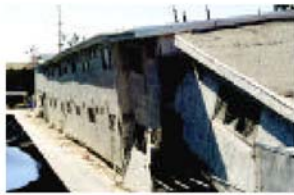
Collapsed woodframe apartment building, Northridge earthquake
