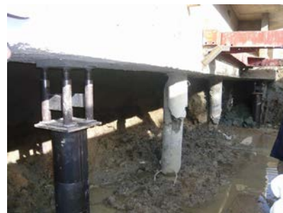
Fig. 24 Structural damage of pile head
