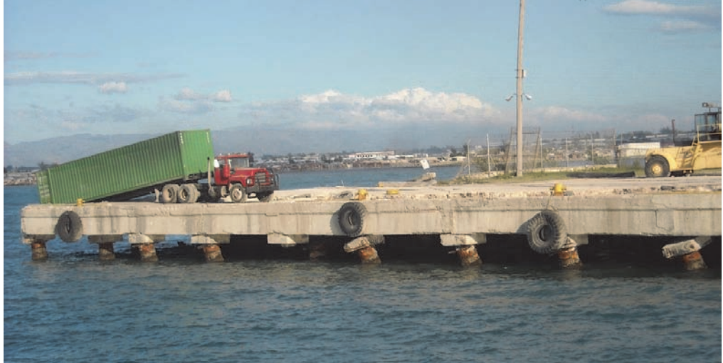
Figure 2-7 Remaining portion of pile-supported pier at the Varreux terminal, Port de Port-au-Prince, following the 2010 Haiti earthquake (Source: Scott Chodkiewicz, U.S. Army Corps of Engineers).
