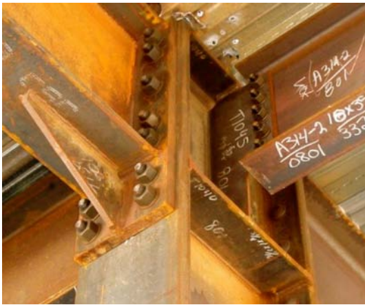
Figure 7-2 - Installed connection continuity plates in a bolted stiffened extended end plate connection.
