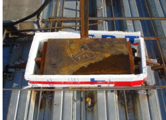
Figure 7-4 - Compressible material used to isolate a protruding bolted stiffened extended end plate connection prior to concrete placement.
