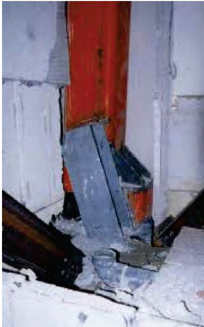
Figure A-29 Retrofit of fractured CJP WCS by welding wide flange studs with stiffened base plates (AIJ, 1995).
