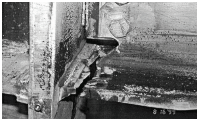
Figure B-13 Typical weak panel zone beam flange failure (Jones et al., 2002).
