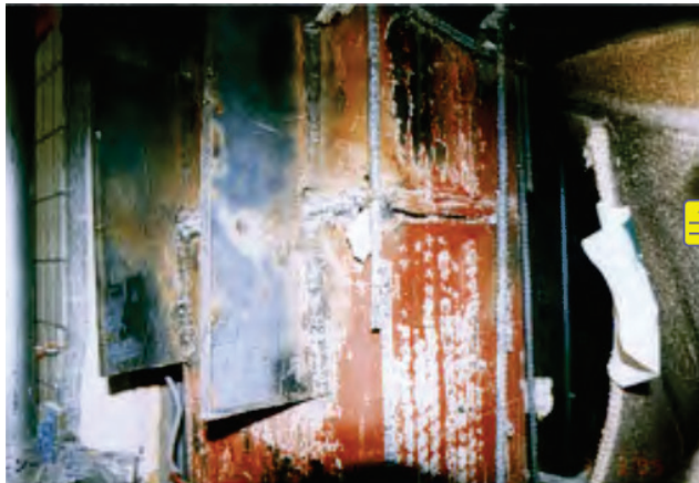
Figure A-27 Retrofit of fractured CJP WCS using welded vertical ribs (AIJ, 1995).
