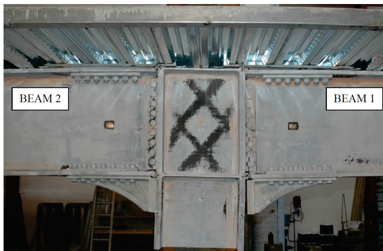
Figure B-30 Doubler plate buckling (Newell and Uang, 2006).
