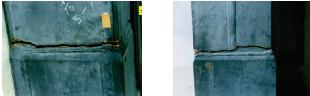
Figure A-14 Fracture of column at welded column splice location (AIJ, 1995).
