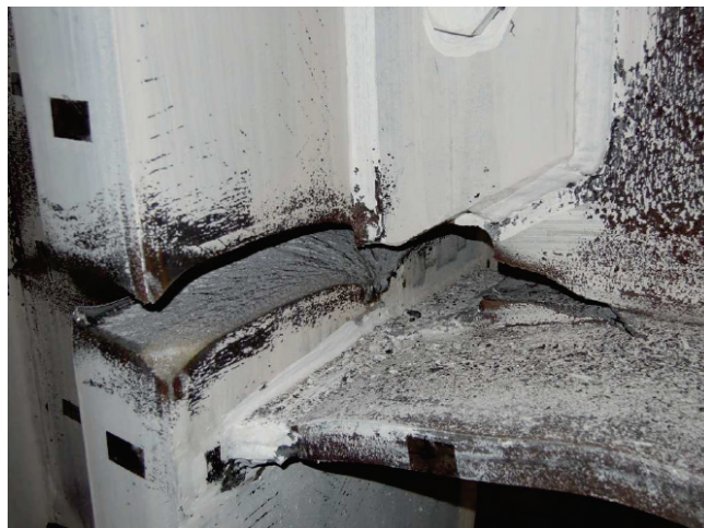
Figure B-27 Column flange fracture (Shin, 2017).
