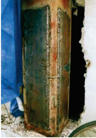
Figure A-28 Retrofit of fractured CJP WCS by welding splice plates on all flanges (AIJ, 1995).
