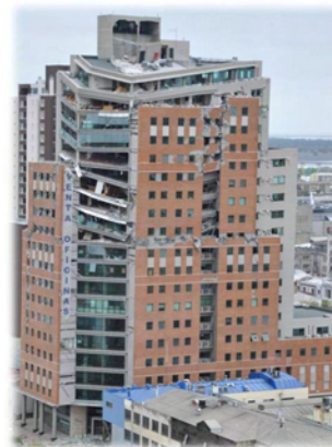
Damage to Torre O'Higgins Building in Concepción, Chile, caused by the magnitude 8.8 earthquake of February 27, 2010. The quake reportedly killed at least 521, injured 12,000, and displaced 800,000 people. 3 Photo courtesy of Jay Harris and Jeff Dragovich, NIST.
